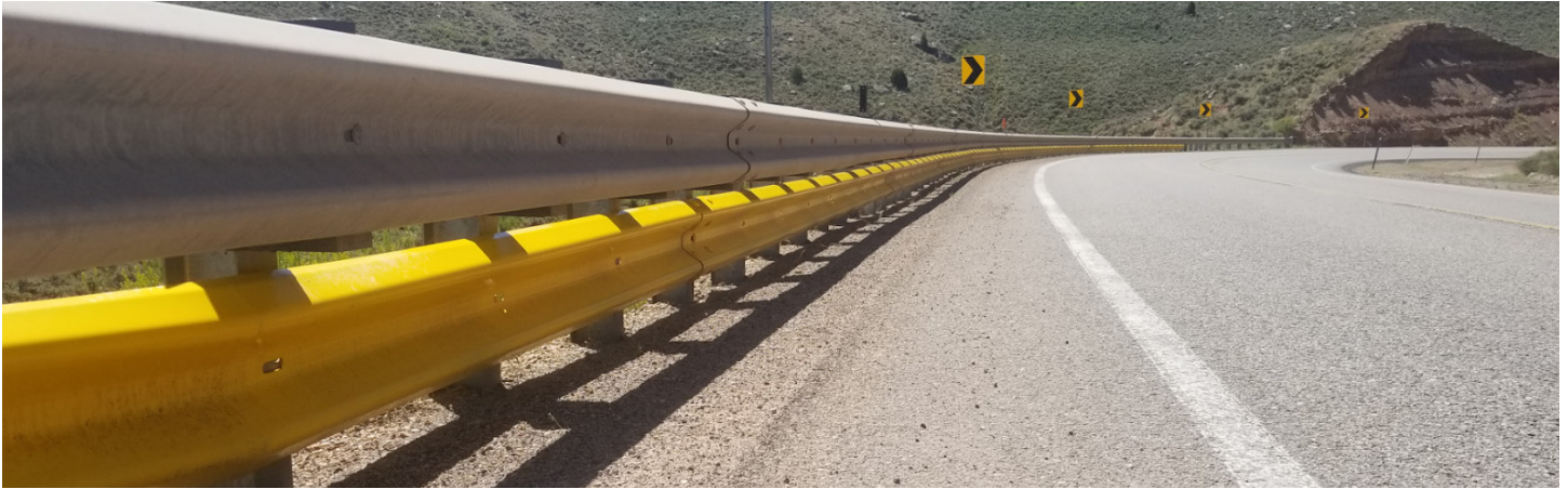
Figure 15. Utah DOT standard W-beam with powder coating.
